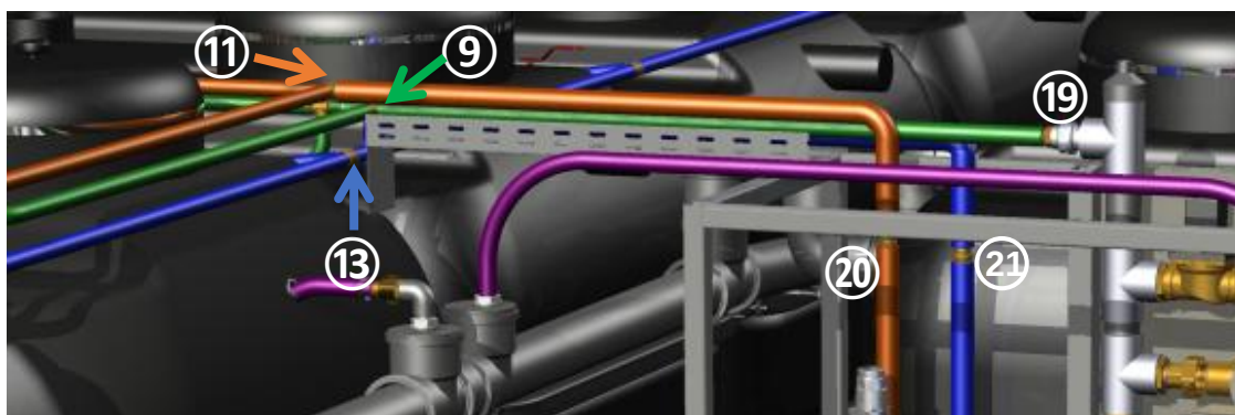
Figure 56: Hose connections between Bioreactor tanks and Technical unit
